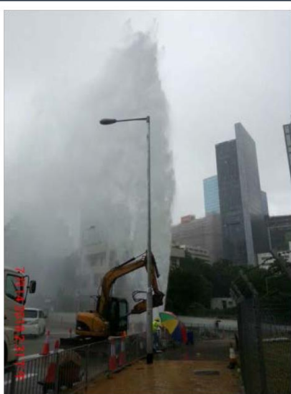
Bursting of WSD dia. 450 mm Fresh Water main
